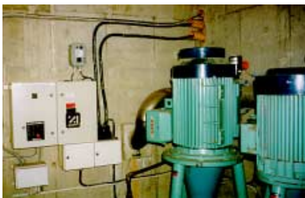
Picture 10.3-1. Control of process water pumps located in a pit some hundred meters from the workshop. Electrical cables leads to the workshop.
