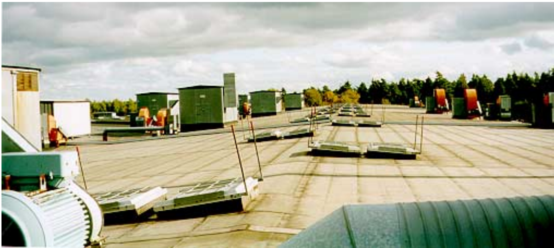
Picture 10.3-3. Extraction fans and equipment for general ventilation or inlet of air on the roof of the workshop. The fans for extraction are showed at the right in end side of the roof.
