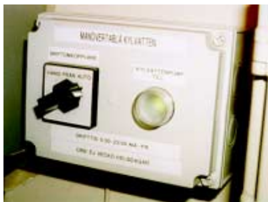
Picture 10.3-2 : Control device in the workshop making it possible to switch off or on the pumps manually or automatically.
