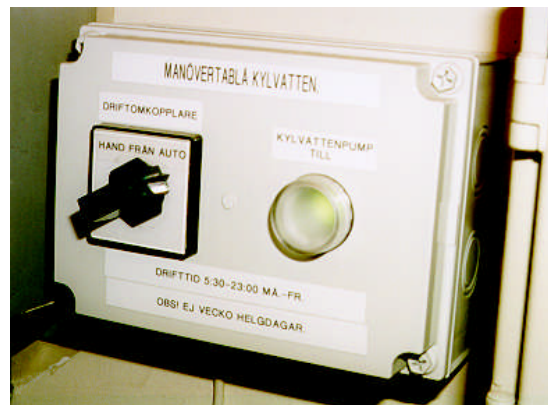
Picture 10.3-2 : Control device in the workshop making it possible to switch off or on the pumps manually or automatically.
