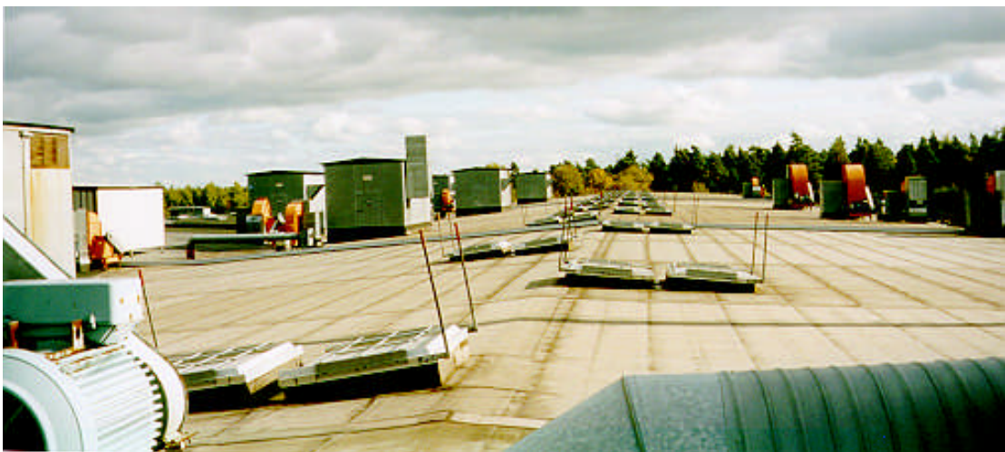
Picture 10.3-3. Extraction fans and equipment for general ventilation or inlet of air on the roof of the workshop. The fans for extraction are showed at the right in end side of the roof.
